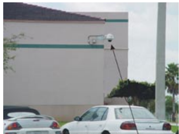
CCTV STRATEGICALLY POSITIONED TO MONITOR VISITOR PARKING AND BUILDING PERIMETER
