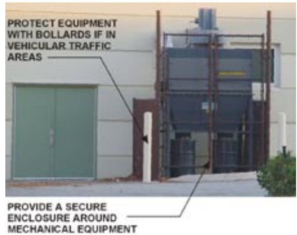
Figure 4.2.3 Mechanical Equipment Example
