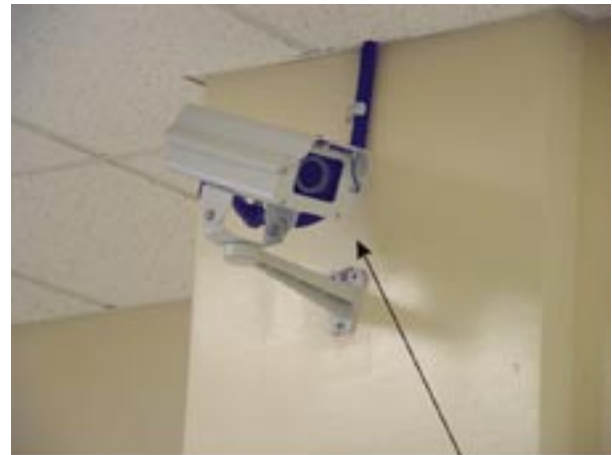
CCTV SHOULD BE INSTALLED IN POTENTIAL PROBLEM AREAS IN NEED OF INCREASED CONTROL
