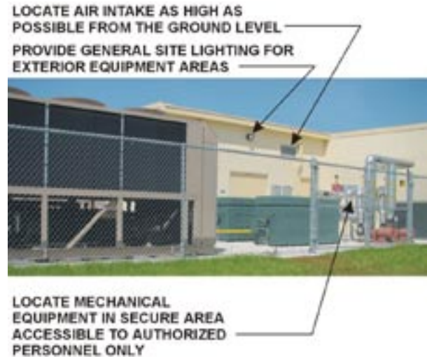
Figure 4.2.1 HVAC/Mechanical Equipment Example
