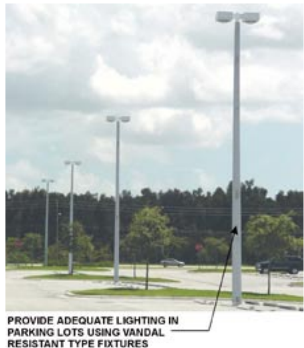
Figure 1.2.6 Parking Lot Lighting
