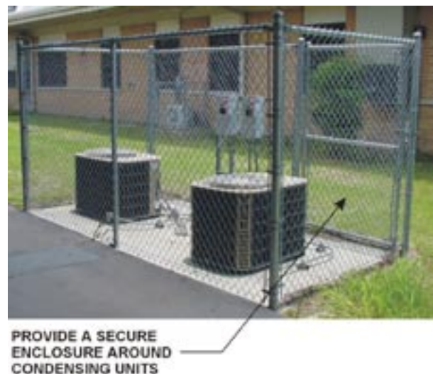
Figure 4.2.2 HVAC Equipment Example
