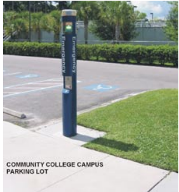
Figure 1.2.7 Provide Blue Light Type Emergency Phones in Community College Campus Parking Lots
